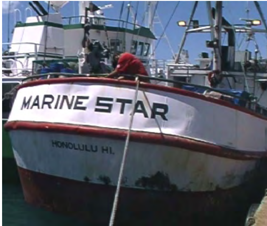
Fig. 8. Work begins on the F/V Marine Star to move the main line shooter from the stern mount.
